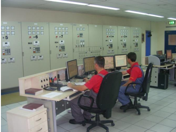
Control room and local panels
