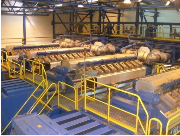
Wartsila Gas Engines
