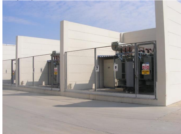
Step up Transformers
